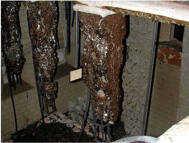
Figure F114. Columns after the first fire test. From the left: A10, C10, D10.
