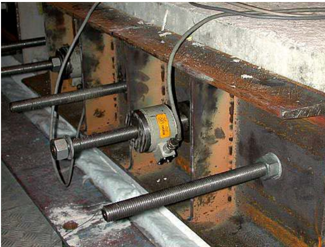
Figure F4. Close-up on load cell.
