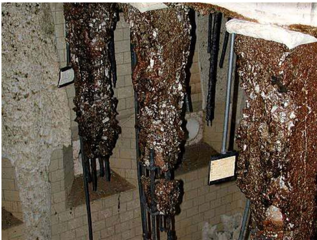
Figure F115. Columns after the first fire test. From the left: A10, C10, D10.
