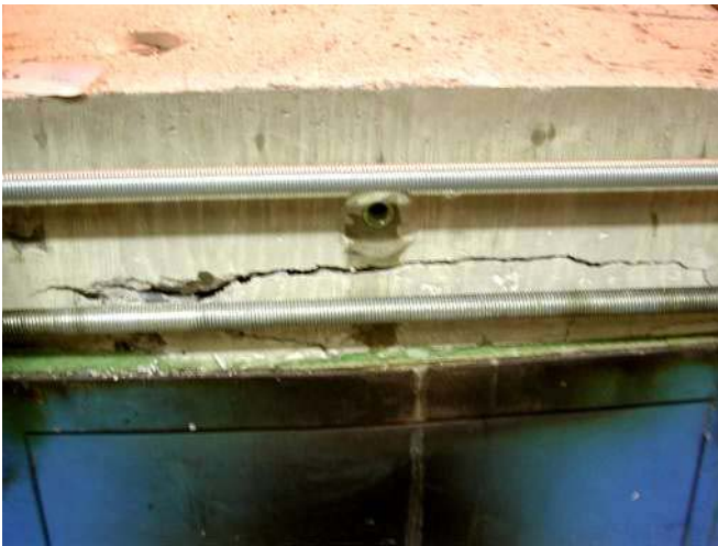
Figure E34. Small slab SS 55 03 during the fire test. A large crack appeared at the edge.
