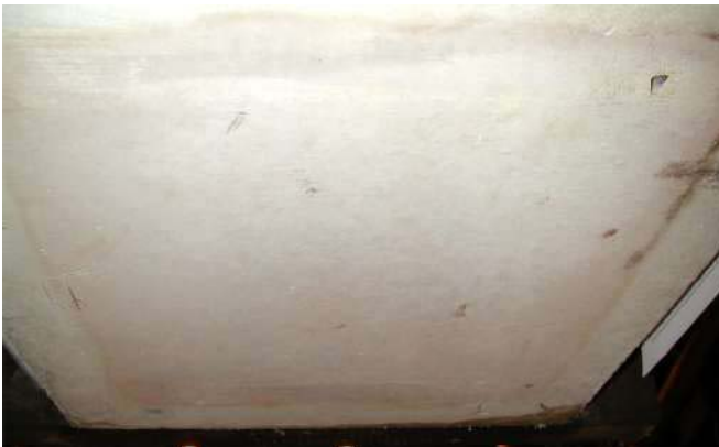
Figure E31. Small slab SS 40 14 after the fire test.
