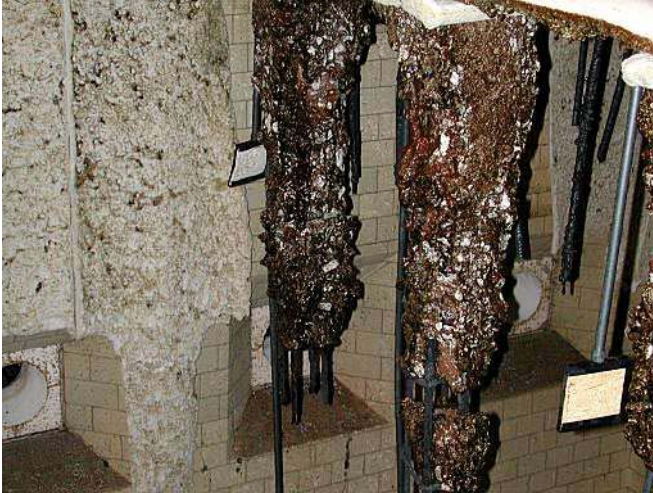
Figure F116. Columns after the first fire test. From the left: A10, C10.
