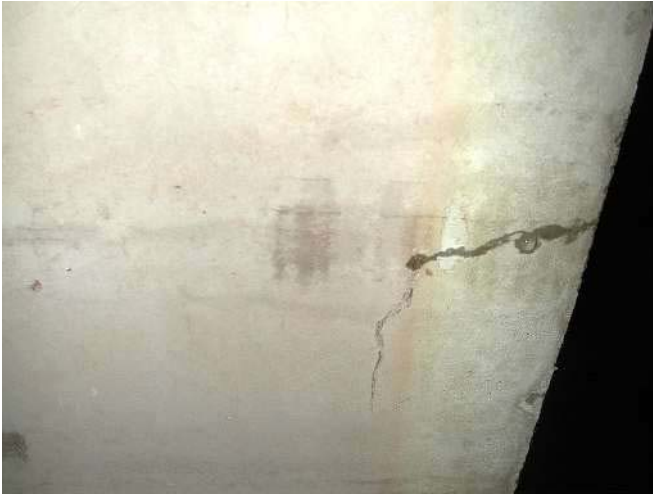
Figure E28. Small slab SS 40 11 after the fire test.
