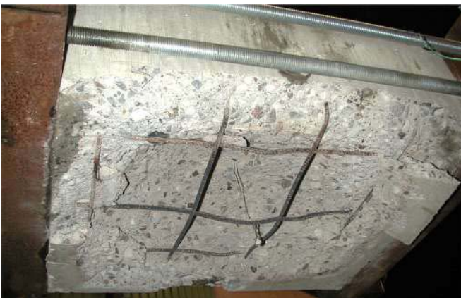
Figure E34. Small slab SS 55 03 after the fire test.
