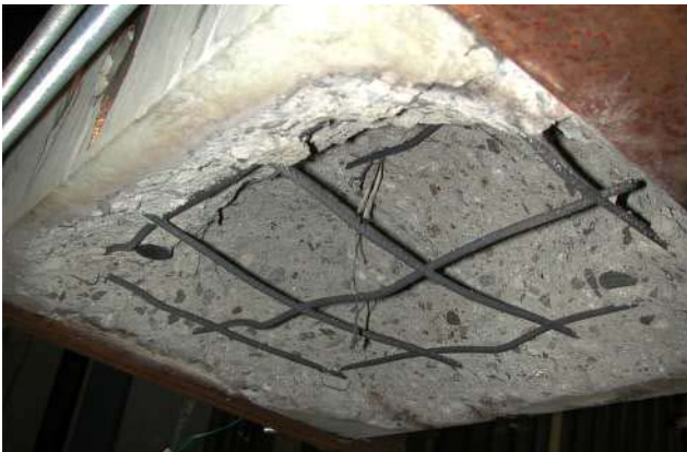
Figure E26. Small slab SS 40 04 after the fire test.
