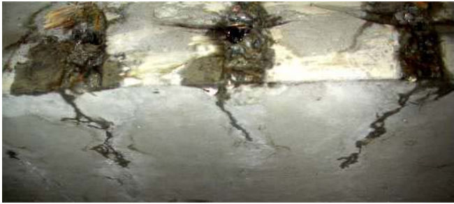
Figure D8. Water pouring out at the pre-stressed wires of a large slab.
