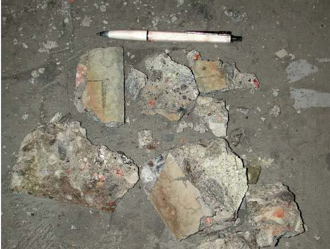
Figure E18. Some of the material that spalled of from SS 30 04.
