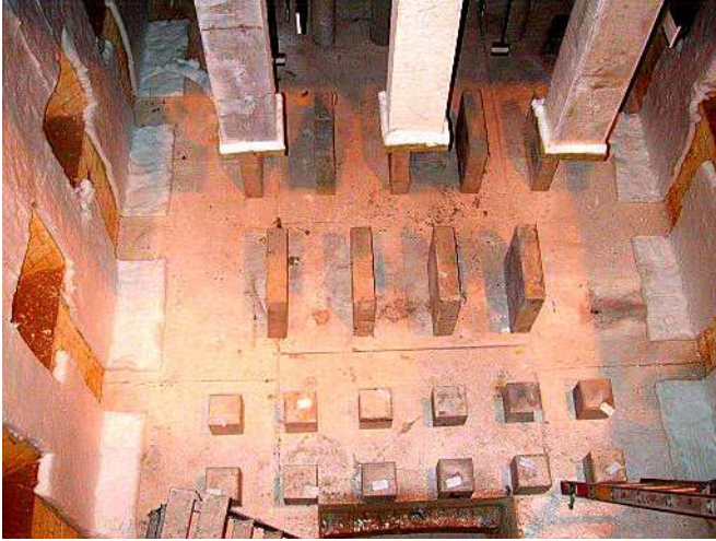
Figure F12. Insulation of furnace walls.
