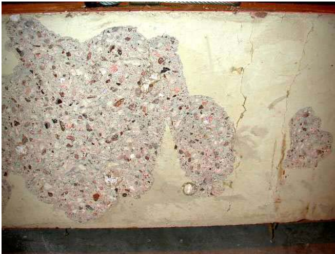
Figure D16. Close-up on beam LB 40 01 after the fire test.
