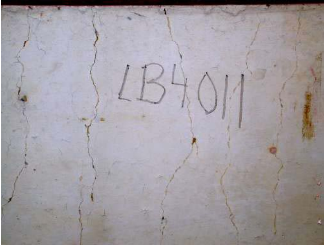
Figure D18. Close-up on beam LB 40 11 after the fire test.
