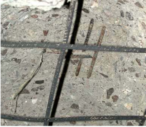
Figure E23. Close-up on small slab SS 40 03 after the fire test.
