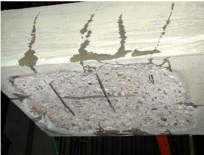
Figure E19. Small slab SS 40 01 after the fire test.
