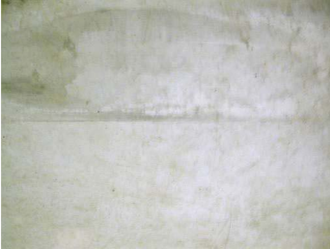
Figure E30. Small slab SS 40 13 after the fire test.
