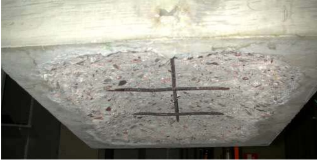
Figure E14. Small slab SS 30 02 after the fire test.
