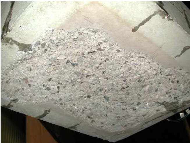
Figure E32. Small slab SS 55 01 after the fire test.
