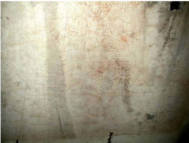
Figure E29. Small slab SS 40 12 after the fire test.
