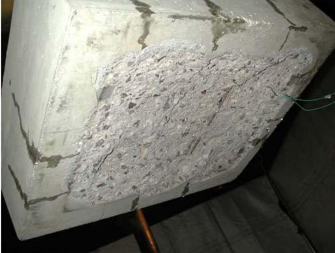
Figure E33. Small slab SS 55 02 after the fire test.
