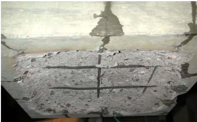
Figure E12. Small slab SS 30 01 after the fire test.
